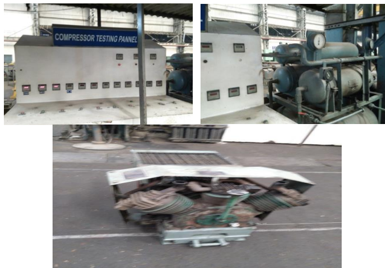
Fig. 4. Compressor Testing Panel, Storage Tank and Reciprocating Air Compressor. [18]
